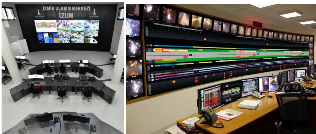
Figure 4.2.14: Example of traffic control centre
