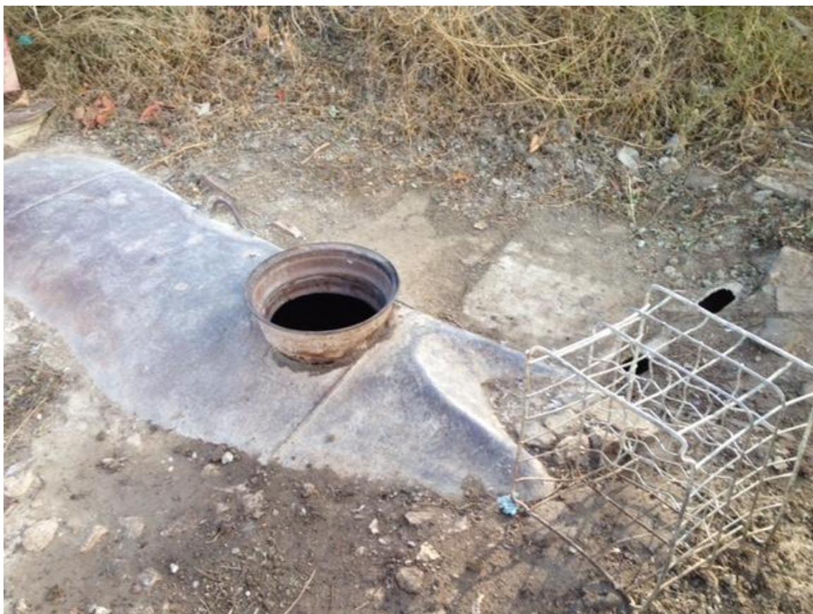
Figure 2-5 Leachate Collection Reservoir
