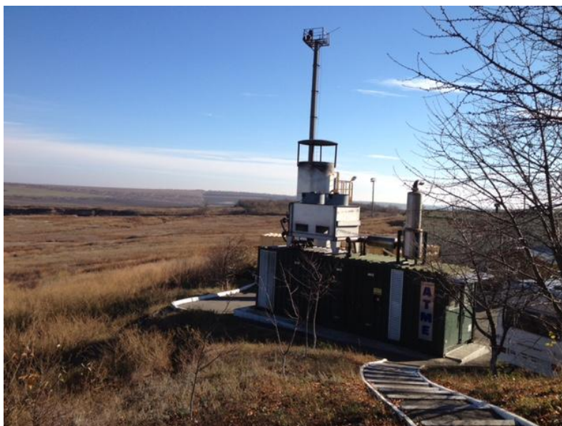
Figure 2-7 Biogas Plant at Tintareni Landfill
