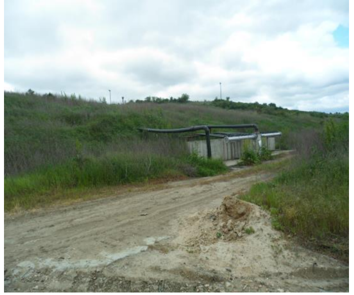
Poor road surface within the site
